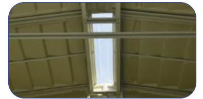
Roof Skylight for natural daylight with DuraMate models
